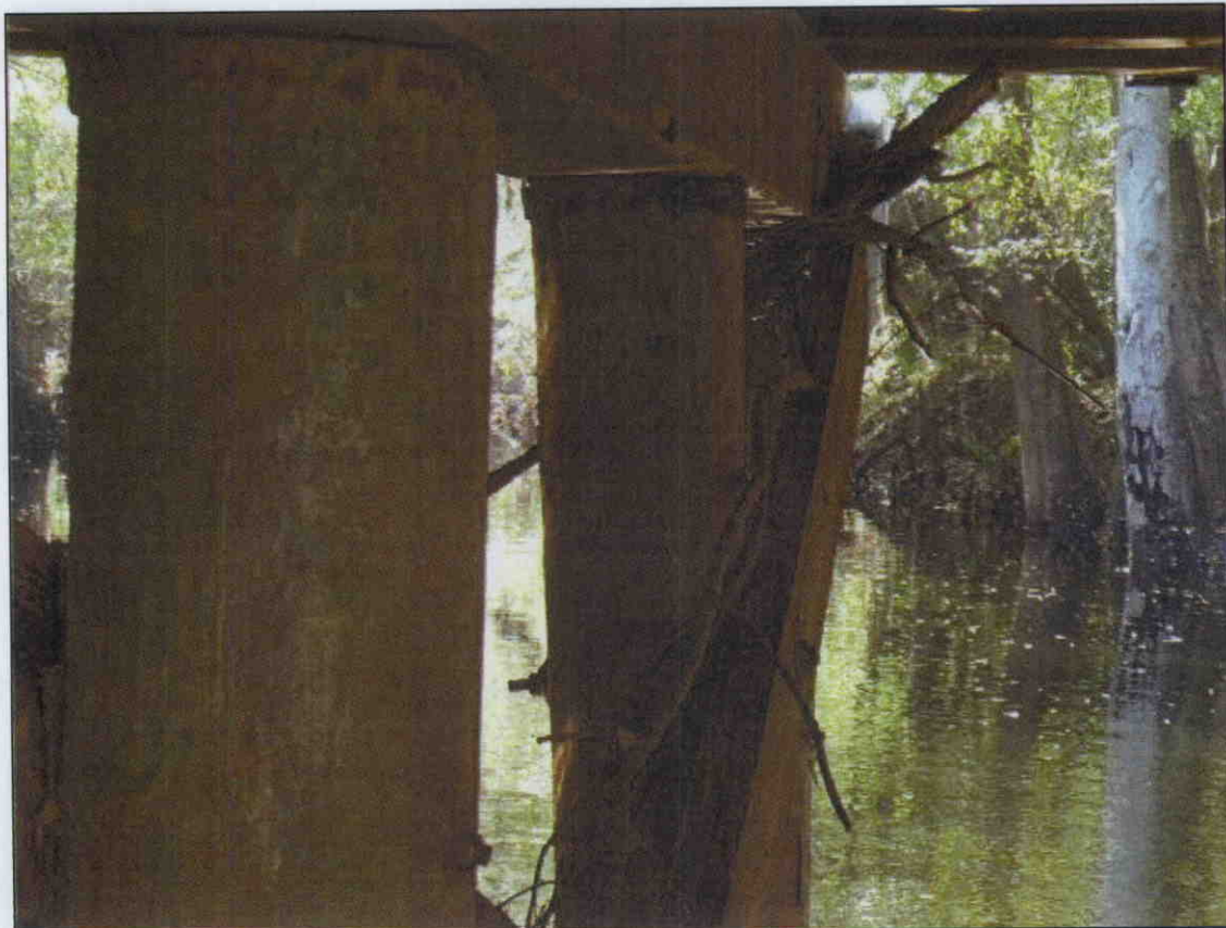
SMALL DRIFT COLLECTING AT BENT 3 SPAN 4 SIDE 3" DIA.
