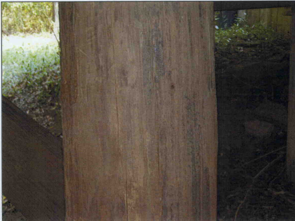
LONGITUDINAL CRACKING ALONG PILES UP TO 1/16" WIDE
