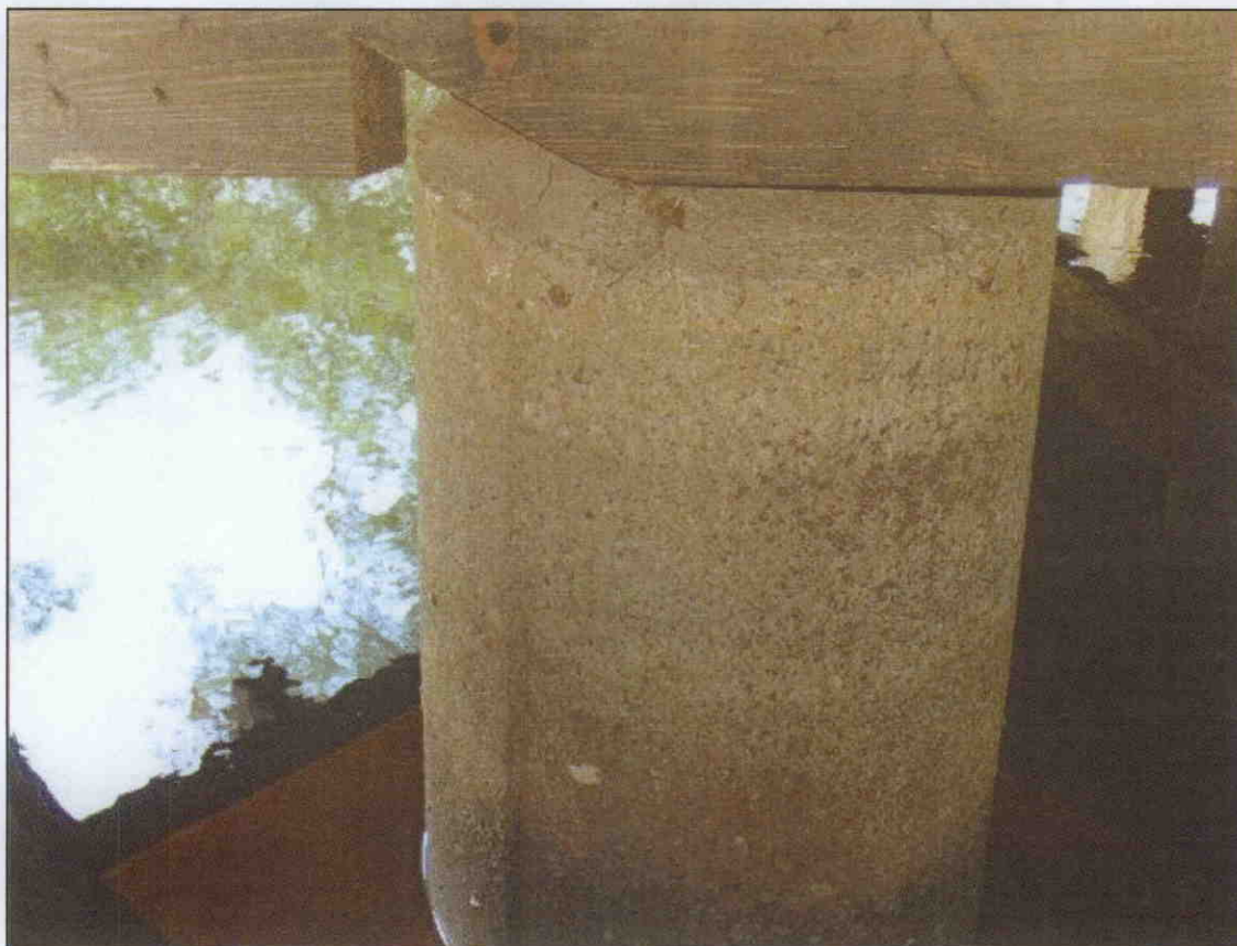
PILE 2 AT BENT 2 ENCASEMENT CRACKED
