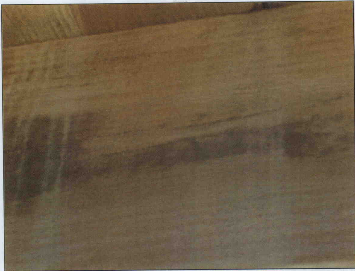
LONGITUDINAL CRACKING ALONG JOIST UP TO 1/16" WIDE
