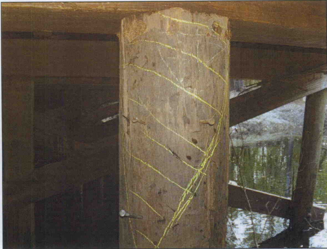
PILE 2 AT BENT 6 NORTH SIDE DECAYED 10" WIDE X 20" HIGH X 3" DEEP
