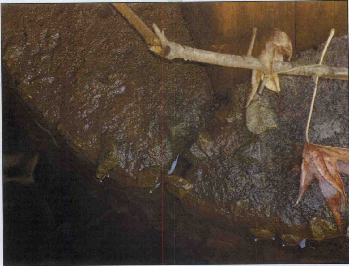
PILE 1 ENCASEMENT AT BENT 4 CRACKED UP TO 1/2" WIDE
