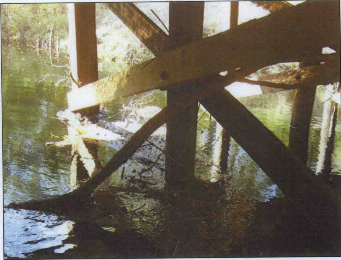
DRIFT COLLECTING AT PILES 1 AND 2 OF BENT 4 UP TO 5" DIA.
