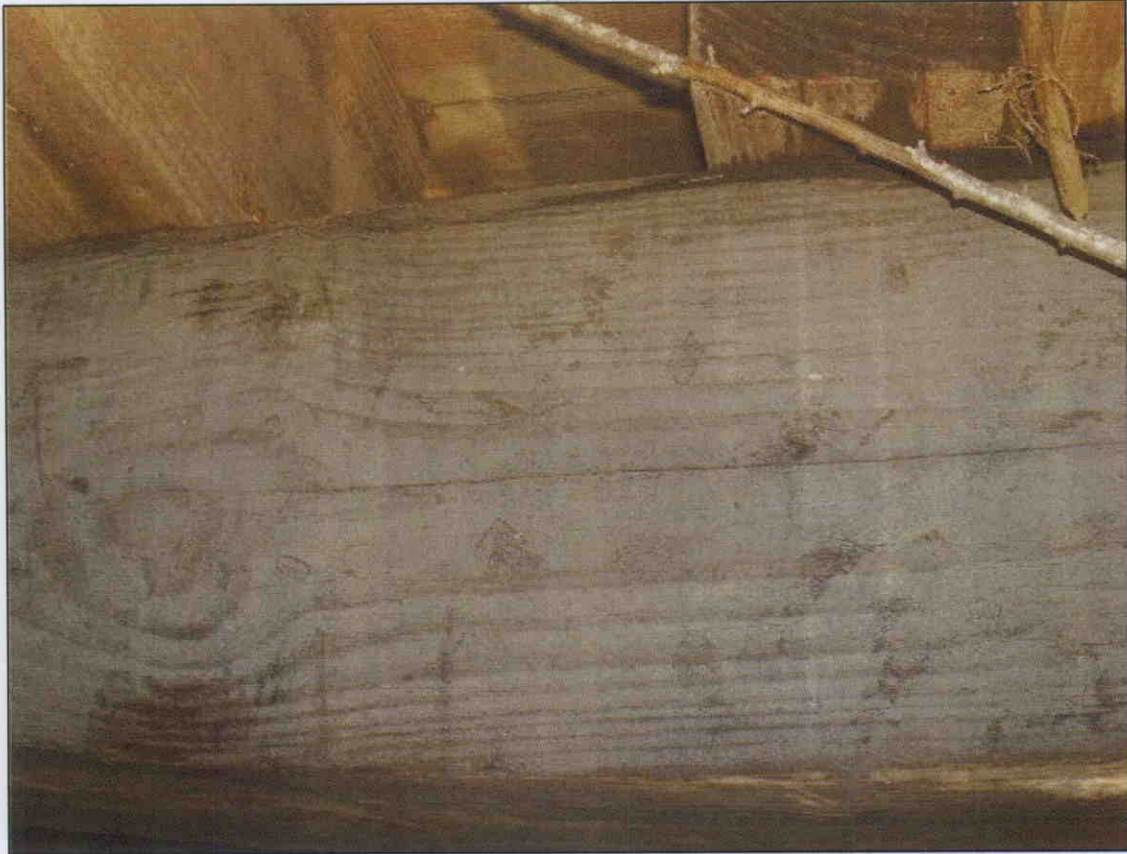
LONGITUDINAL CRACKING ALONG CAPS UP TO 1/16" WIDE
