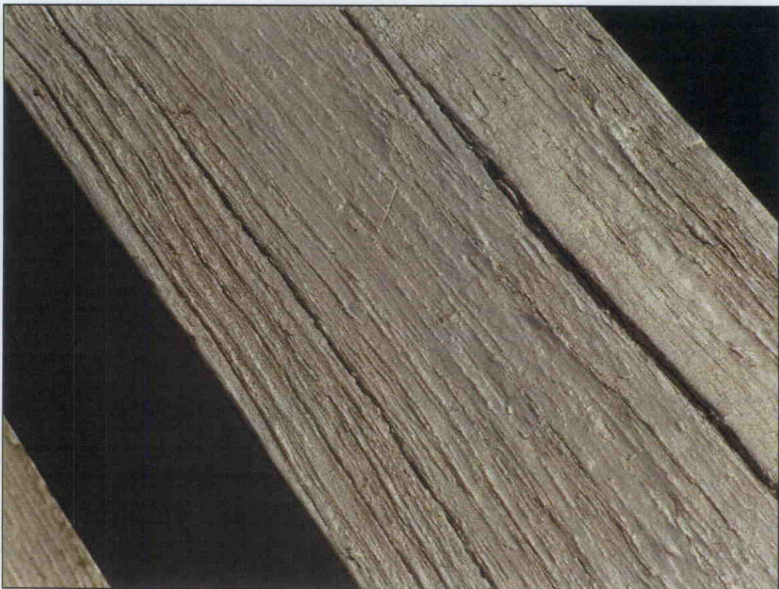
LONGITUDINAL CRACKING IN RAIL BOARDS UP TO 1/8" WIDE
