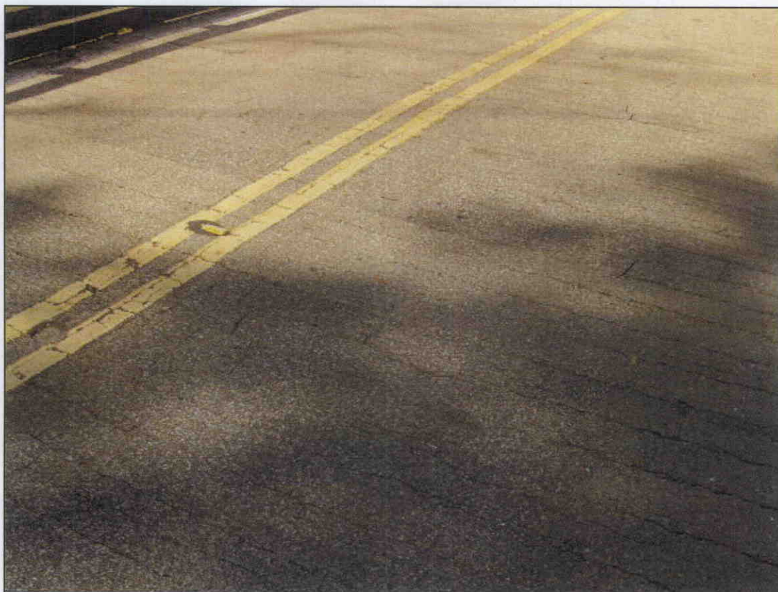
LONGITUDINAL CRACKING/TRANSVERSE CRACKING IN ASPHALT WEARING SURFACE IN ALL SPANS
