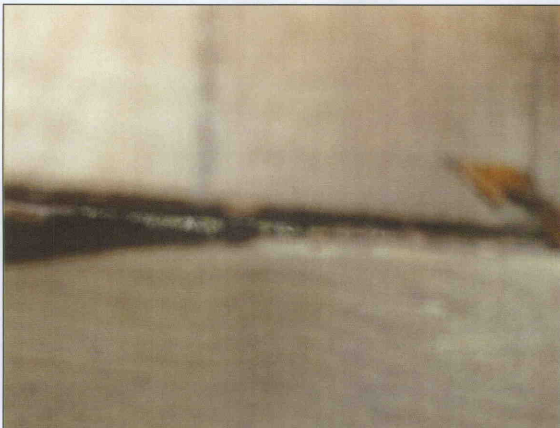
JOIST 1 IN SPAN 1 OVER BENT 1 3/16" GAP BETWEEN JOIST AND CAP, JOIST 2 SIMILAR.
