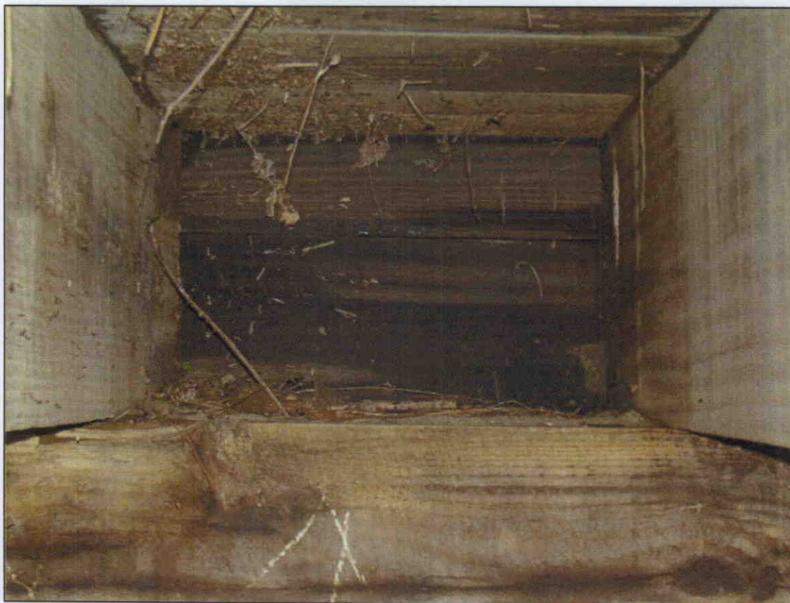
SIGNS OF BULKHEAD LEAKAGE ALONG TOP OF END BENT CAPS
