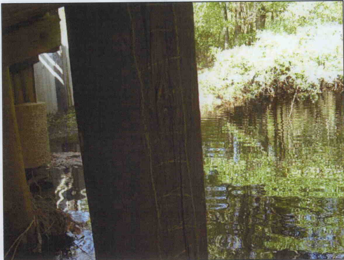
PILE 3 AT BENT 4 SOUTH SIDE DECAYED/SPLIT 3" WIDE X 30" HIGH X 2" DEEP
