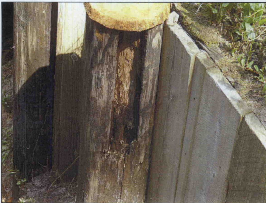
SOUTHWEST WINGPILE DECAYED AND HOLLOW
