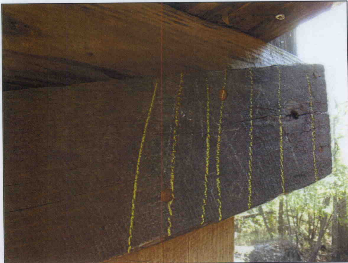
CROSSBRACE AT BENT 4 SPAN 5 SIDE DECAYED 2' LONG
