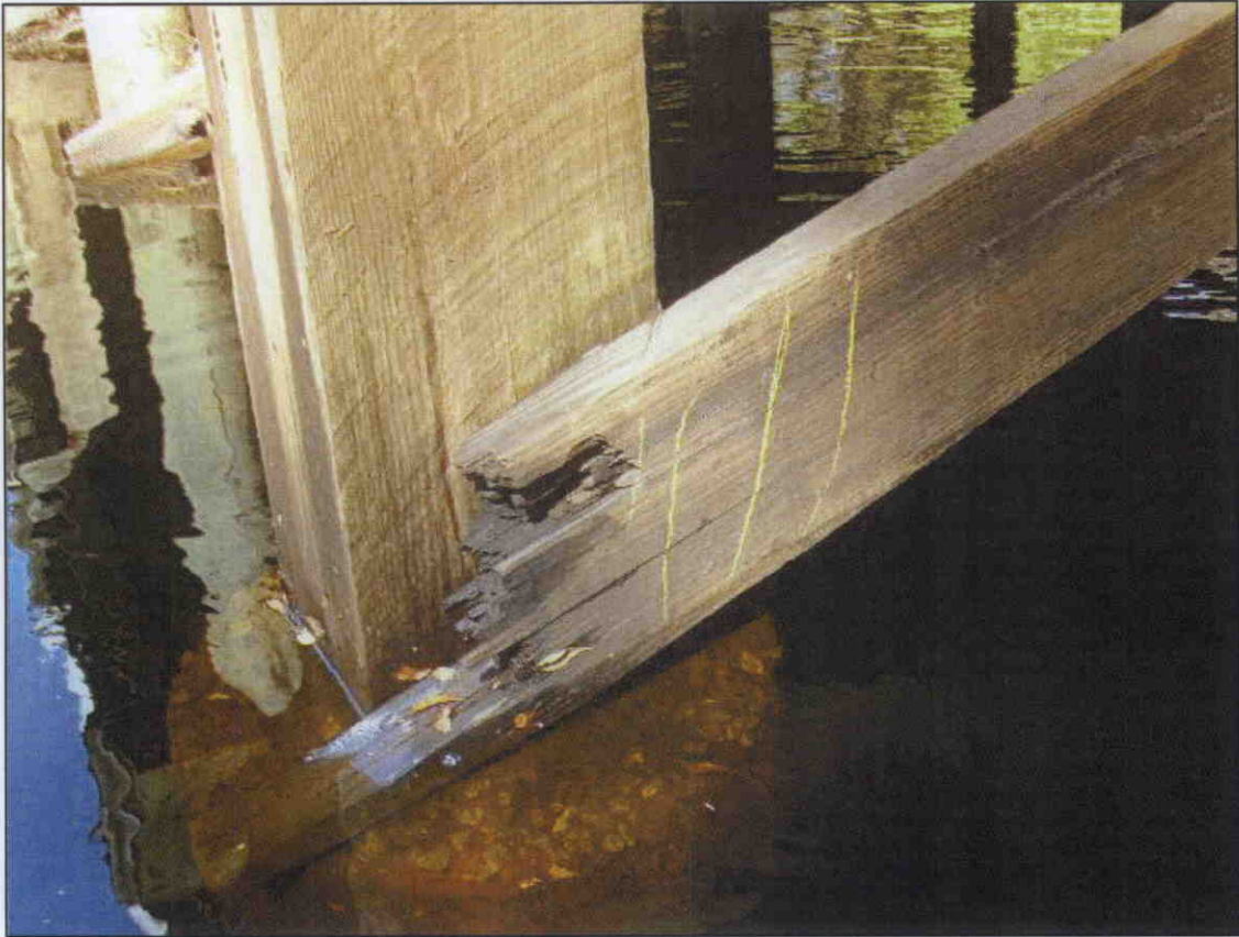
CROSSBRACE AT AT BENT 2 SPAN 2 SIDE DECAYED AT PILE 1 , 2' LONG.
