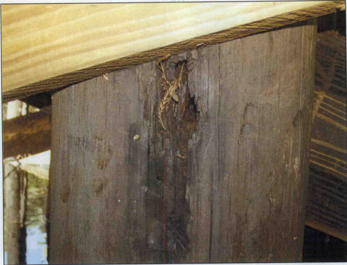
PILE 2 AT BENT 4 DECAYED AT BOLT HOLE 1" WIDE X 4" HIGH X 10" DEEP
