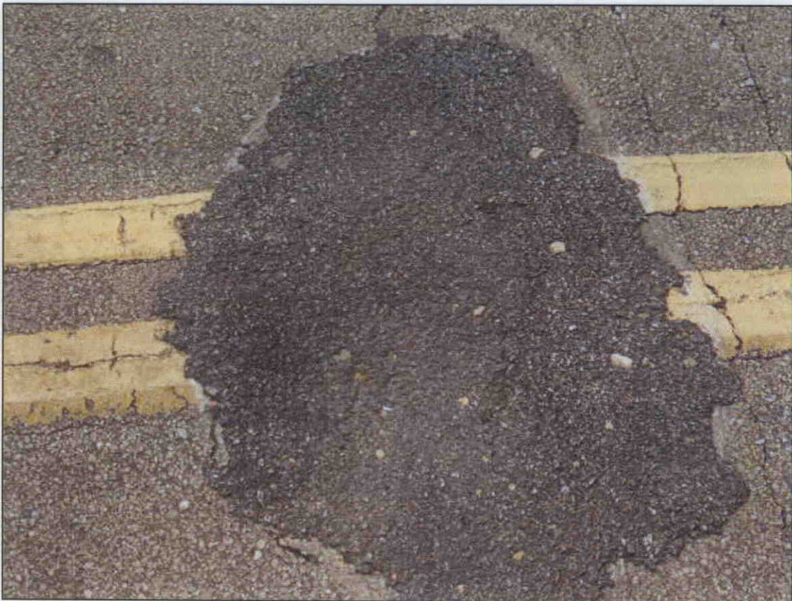
SETTLED AREA AT CENTERLINE OF SOUTH APPROACH 2' WIDE X 16" LONG X 3" DEEP
