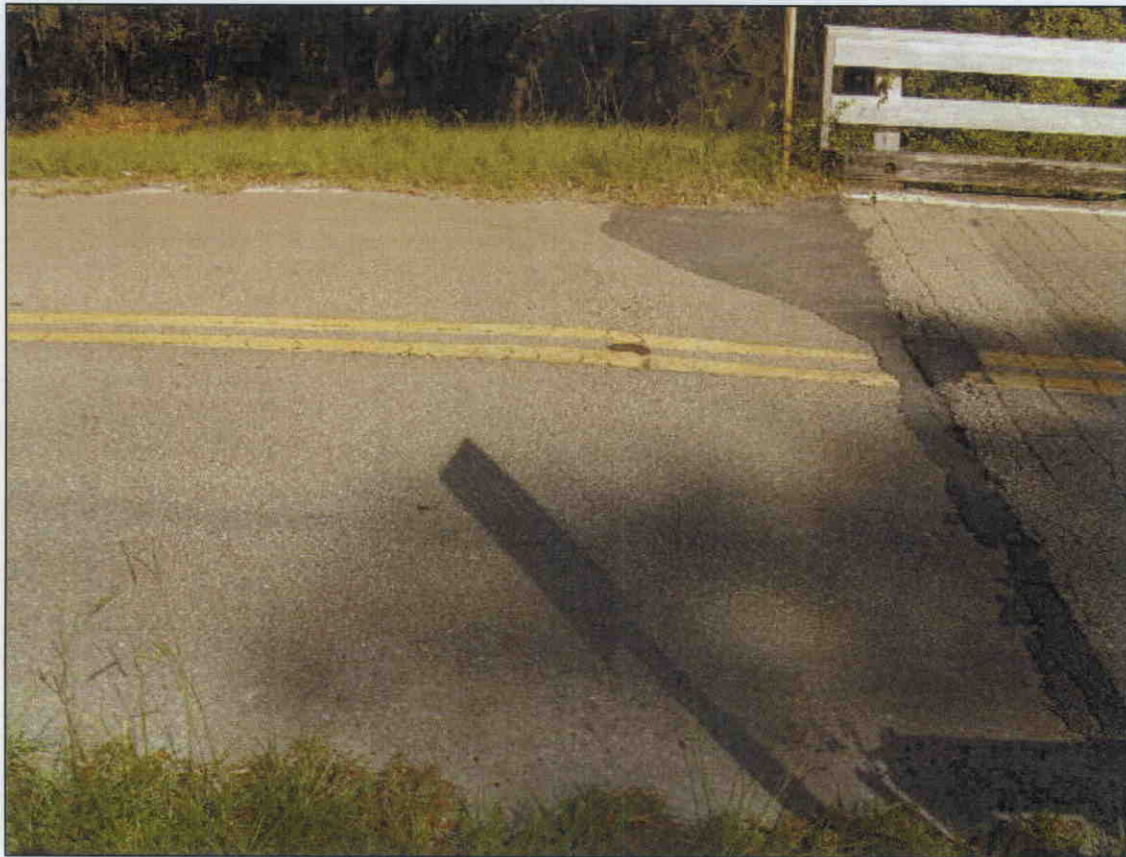
NORTH APPROACH ASPHALT WEARING SURFACE SETTLED UP TO 2"
