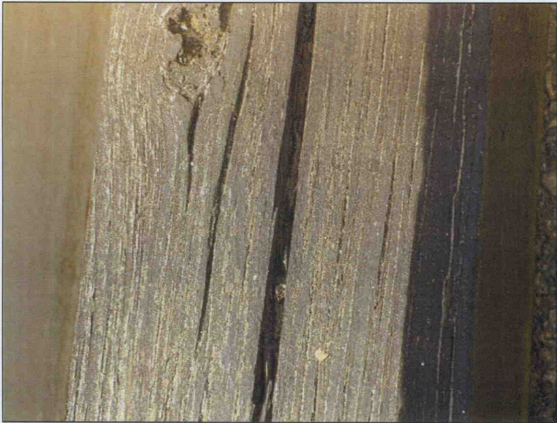
LONGITUDINAL CRACKING IN WHEEL GUARDS UP TO 1/4" WIDE
