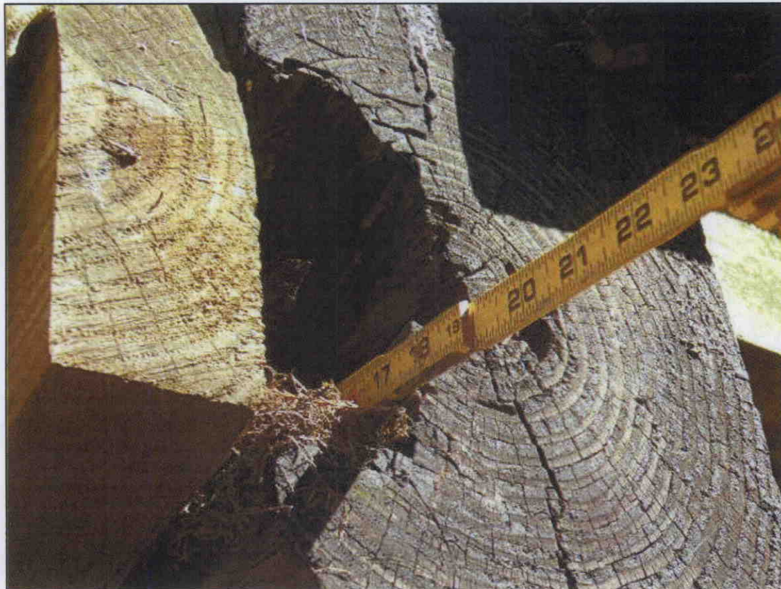
WEST END OF BENT 2 CAP DECAYED 4" WIDE X 6" HIGH X 17" LONG
