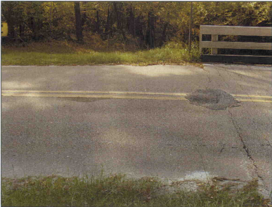
SOUTH APPROACH ASPHALT WEARING SURFACE CRACKED AND SETTLED 1"
